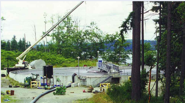
BOISE CASCADE - Pumping sludge 2000 feet from the bottom of an active clarifier
